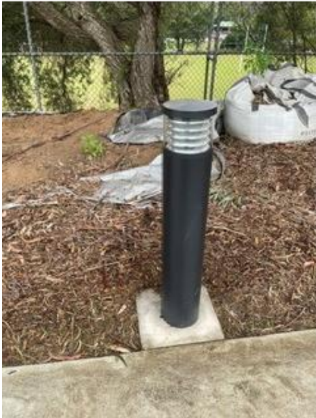
Photo 1: Completed pathway lighting
